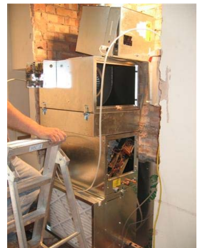
The air sourced heat pump is installed
